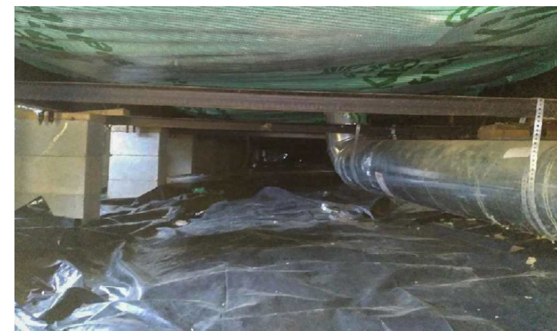
Damaged or disconnected ducts allow the air you pay to heat escape under the home.
